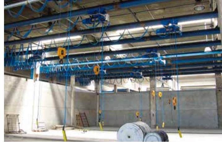
Magazzino trasporto coils - Coils transport warehouse
