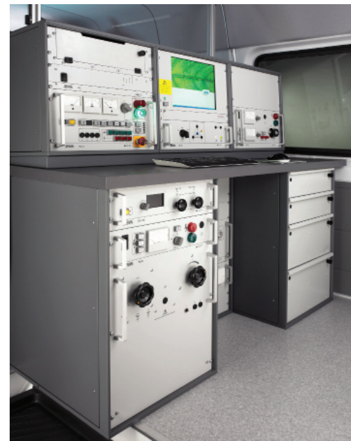
IRG 3000, integrated in the cable test van
