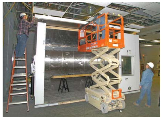
ESPEC will come to your site for assembly of the system, start-up, and operator training.
