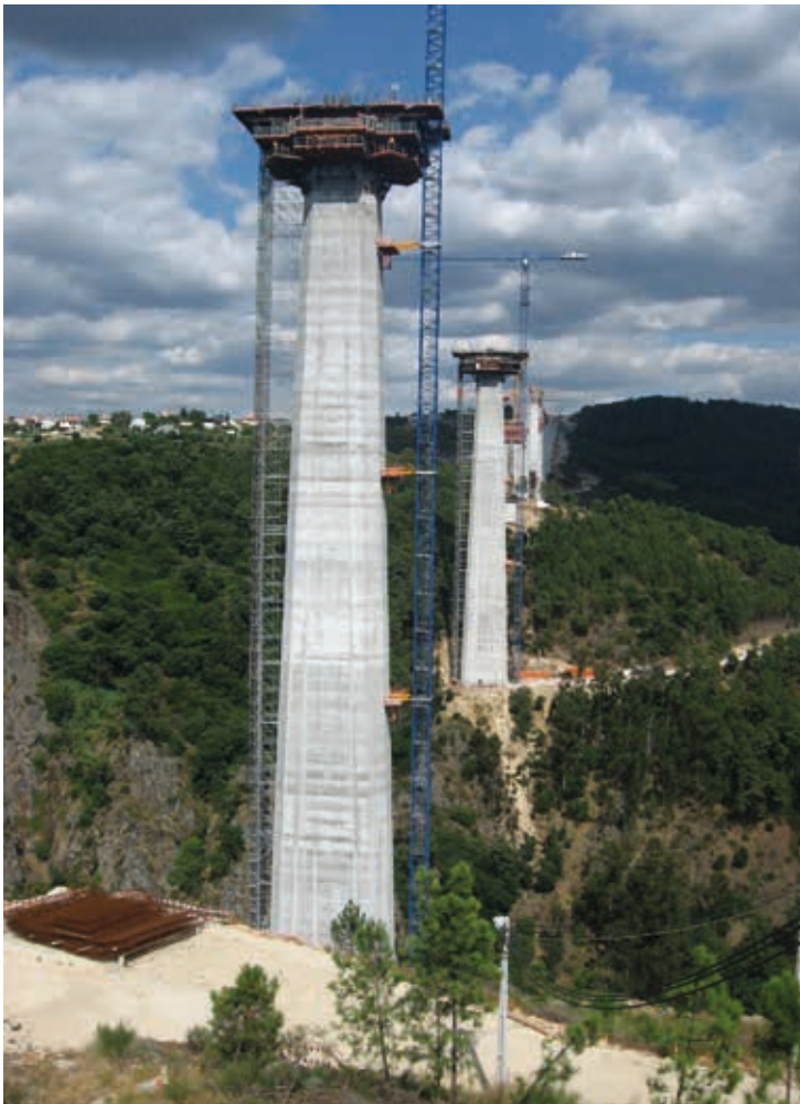
Construction of pier segment on pier at great height. Access with BRIO stair
