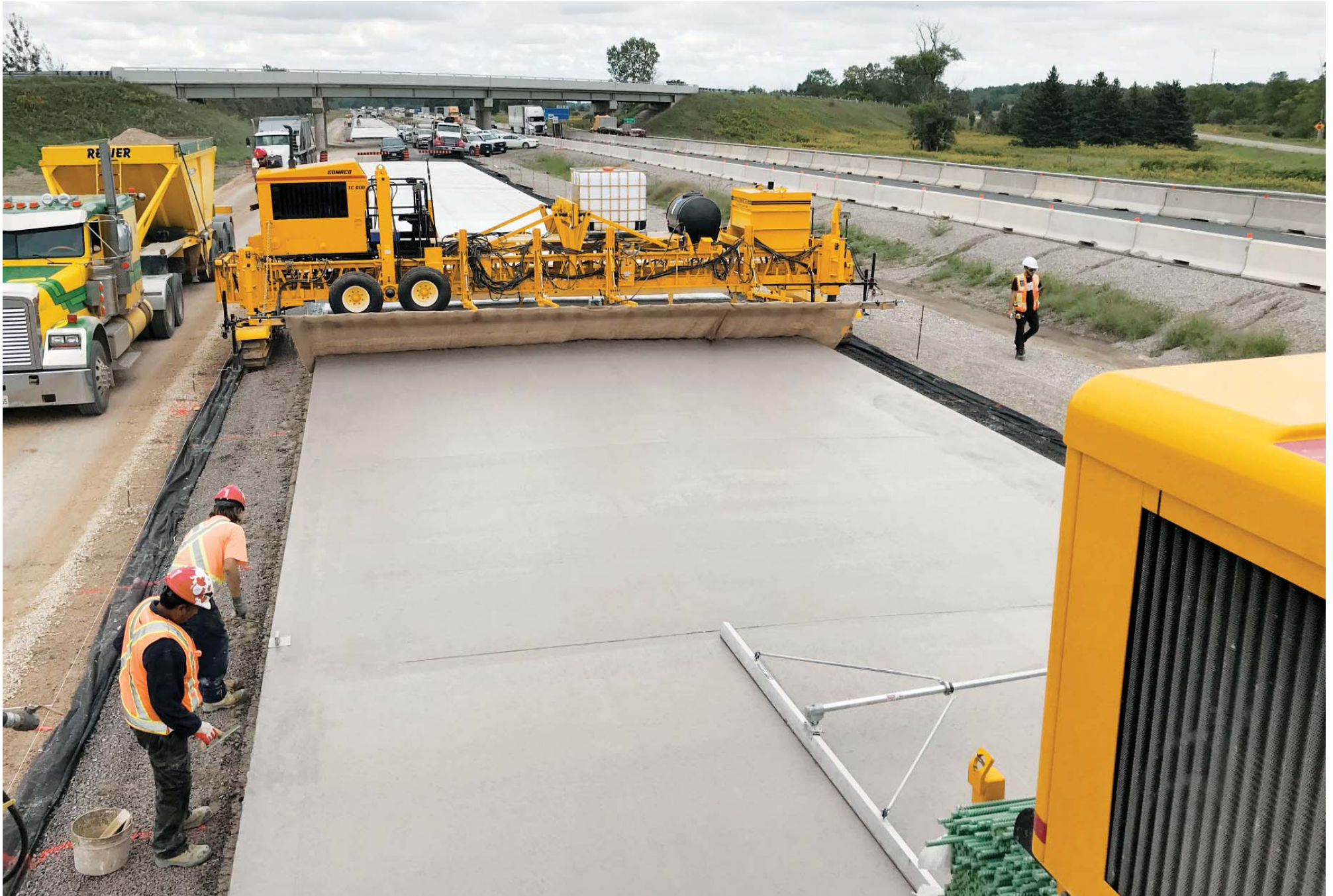
A burlap drag was added to this T/C-600 texture/cure machine to give the highway project the required texture before applying the cure.
