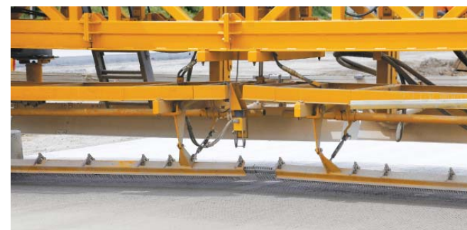
Longitudinal tining with a sonic sensor mounted over the center of the slab.
