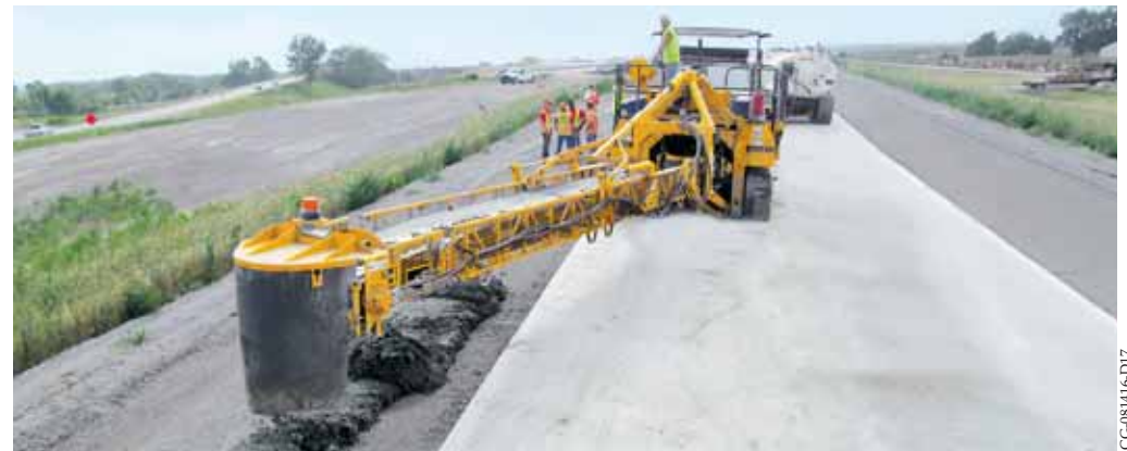
Placing accuracy with the discharge conveyor is accomplished with joystick control next to the operator's chair.
