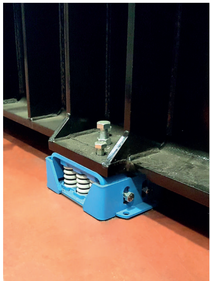
Generator set insulated with VIBRABSORBER+Sylomer®
