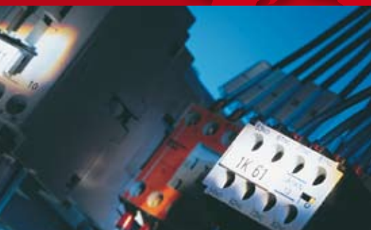
Control gear and equipment location labelling
