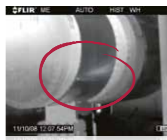
Gas leak in a petrochemical plant
