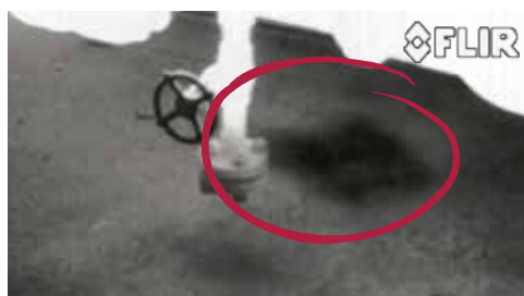
Captured gas leak from production site.
