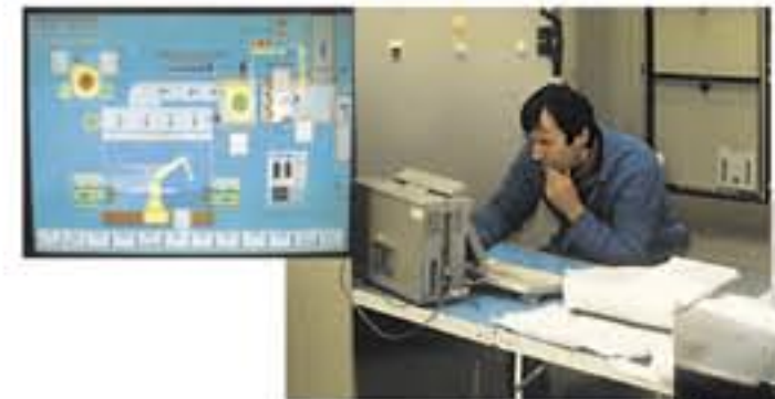
▲ AMC - Technician controlling an automated system
