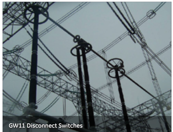
GW11 Disconnect Switches
