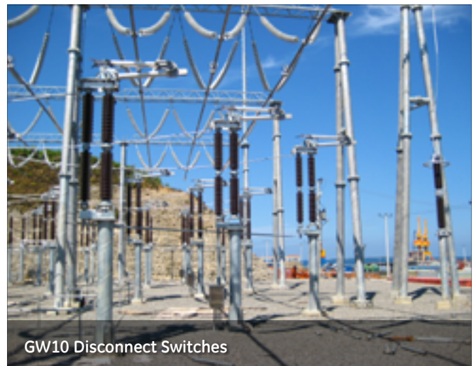
GW10 Disconnect Switches
