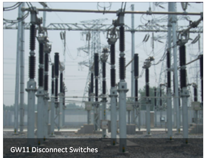
GW11 Disconnect Switches
