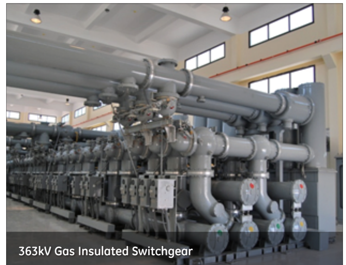
363kV Gas Insulated Switchgear at Golmud Substation
