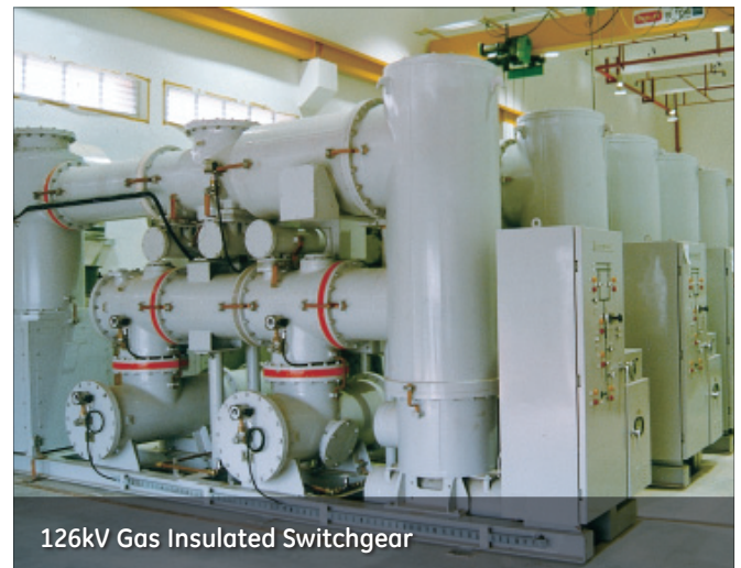
126kV Gas Insulated Switchgear
