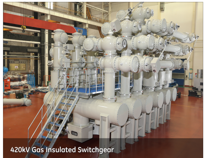
420kV Gas Insulated Switchgear
