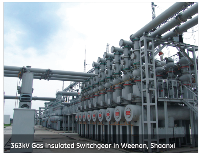
363kV Gas Insulated Switchgear
