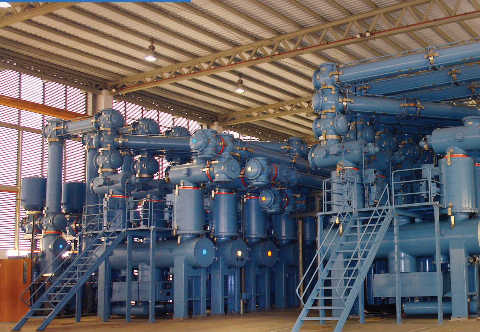
420kV Gas Insulated Switchgear
