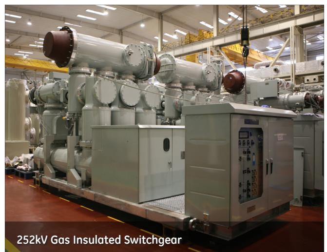
252kV Gas Insulated Switchgear
