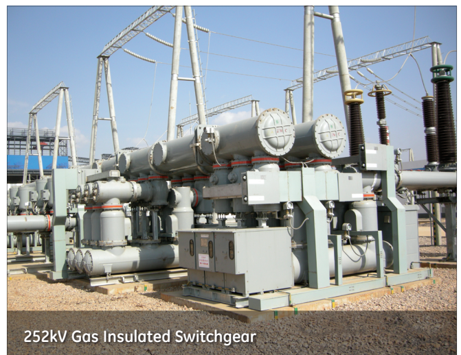
252kV Gas Insulated Switchgear
