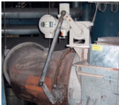
New actuator on existing valve
