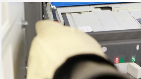
Screws Help Secure The Breaker
