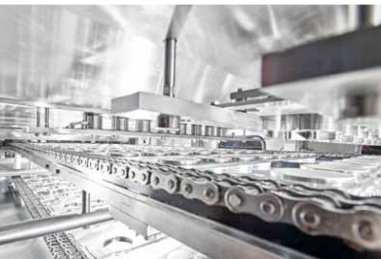
The view of the tunnel clearly shows the newly designed hygiene zone – the tunnel is clean!
