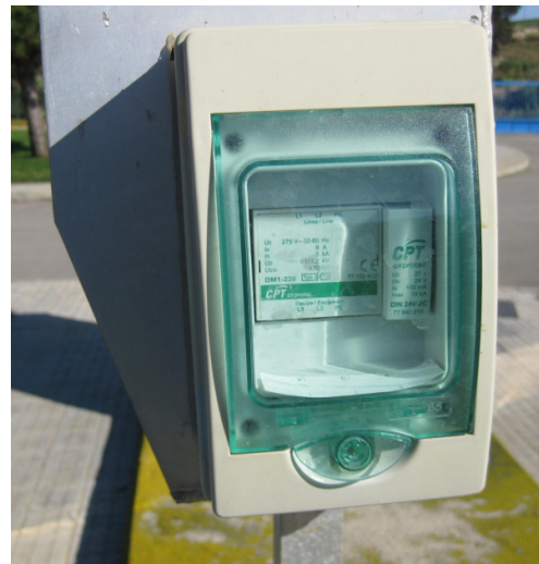
Fig. 6. Field device solution, comprised of data network protection and electrical supply surge protection with EMI filter
