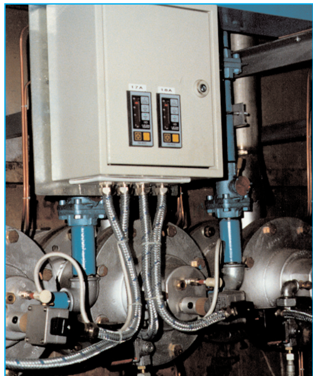
Copper tube heat treat furnace with recuperative, radiant burners, model SER (Europa Metalli)
