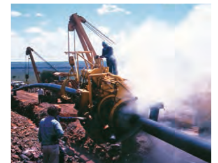
◇ Pipeline in Kenya (1978)
