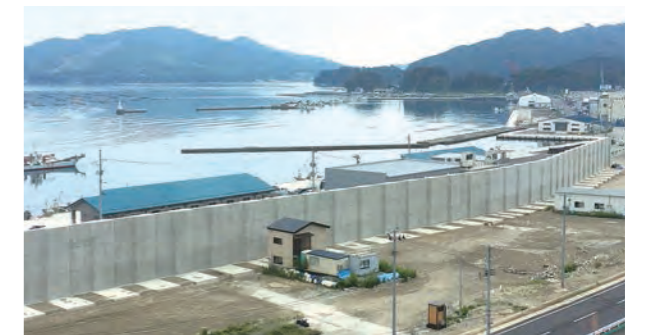
◇ Yamada Fishing Port Hybrid Tide Embankment (Iwate Pref.) / On-site construction work was minimized by precasting the embankment blocks in the factory in advance.
