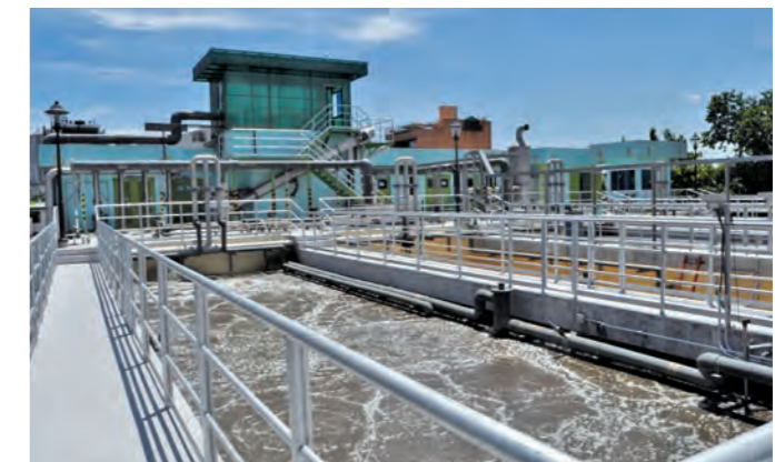
◇ Poblacion Sewage Treatment Plant (Philippines)
