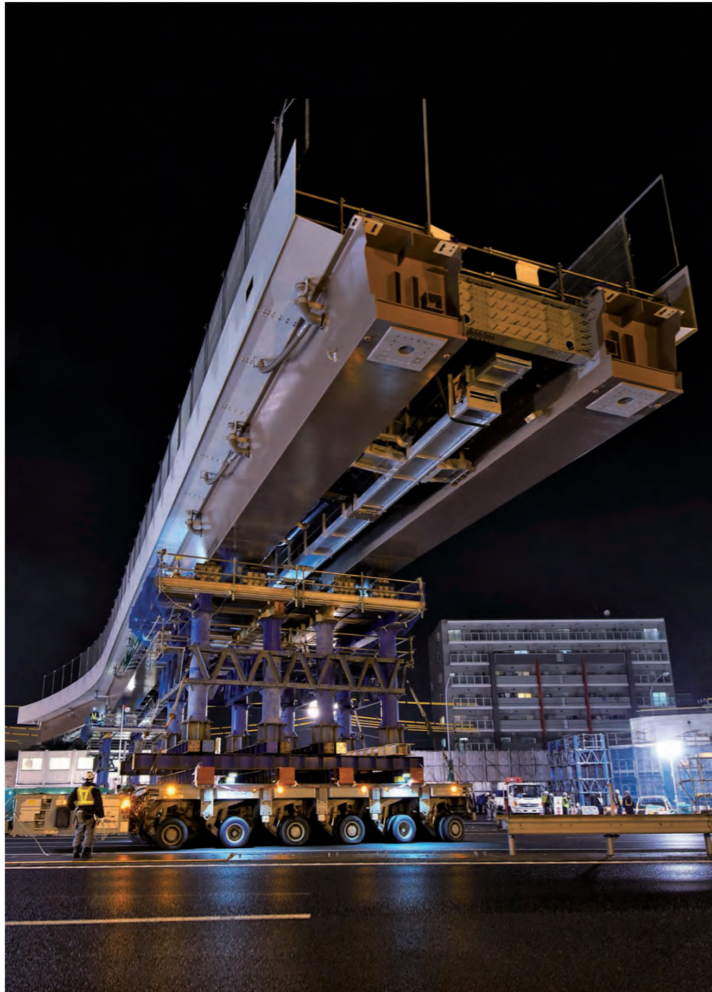
◇ Onitaka Parking Area bridge erection work (Chiba Pref.) / The bridge was fabricated with millimeter accuracy, and erection was completed in 3 hours at night.
