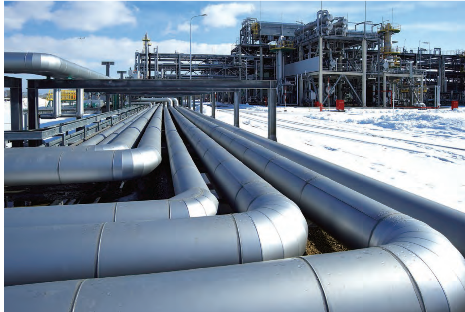
◇ Yufutsu Natural Gas Plant (Hokkaido) / Realizing stable energy supply by treating natural gas extracted from several thousands meters below the surface.
