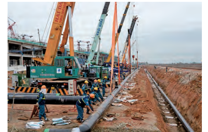
◇ Noi Bai International Airport fueling equipment (Vietnam)
