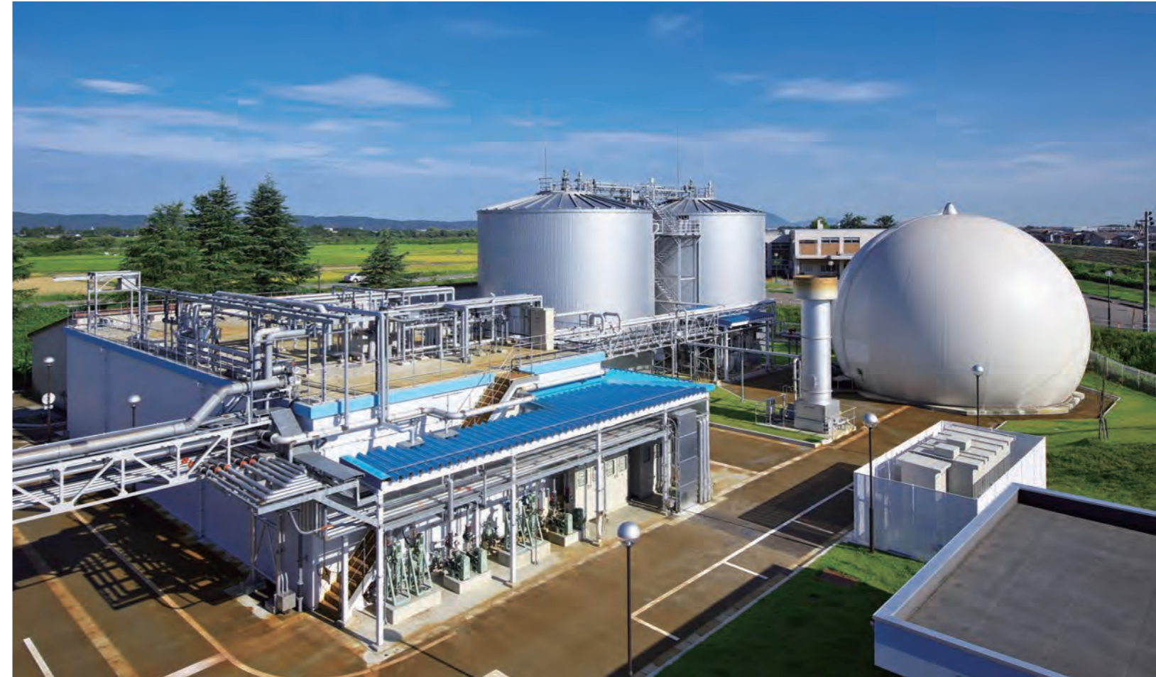
◇ Biomass power generation from kitchen waste (Niigata Pref.) / Collected kitchen waste is fermented, producing biogas for use in power generation.
