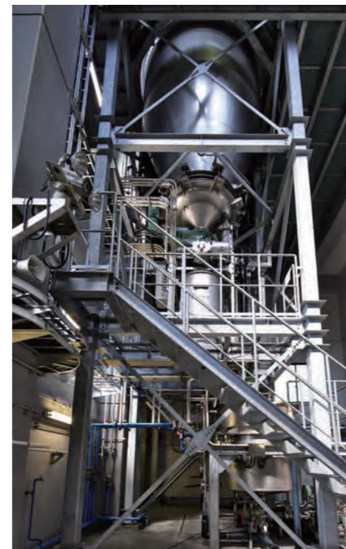
◇ Activated carbon powder injection equipment / Components that cause bad odor, etc. are removed, creating delicious water.
