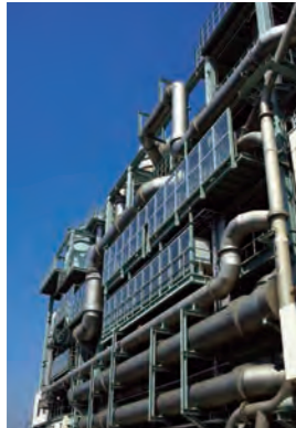
◇ Sludge incinerator that reduces generation of greenhouse gases (GHG) by high temperature incineration of sewage sludge at 850°C or higher
