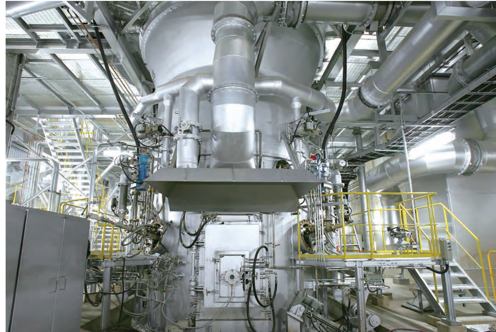
◇ Clean-Hill Homan Gasification and Melting Furnace (Fukuoka Pref.) / Facility where wastes are gasified and melted at high temperature, and are converted into slag, metal and other resources that can be utilized effectively.
