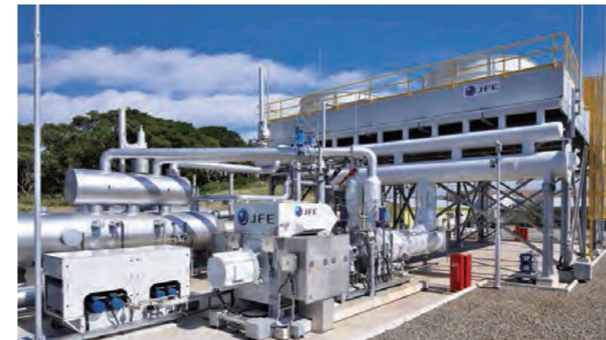
◇ Medipolis Ibusuki Geothermal Power Plant (Kagoshima Pref.)
