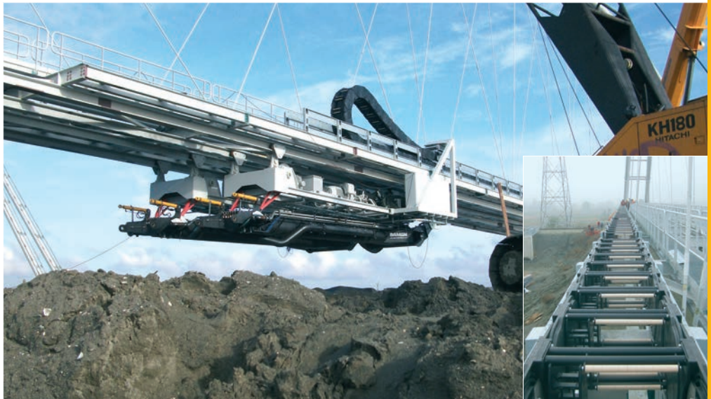
Cleaning of a port basin in Antwerp. On a stroke of 138 meters an e-chain® Series E4.350 guides cables and hoses with a total additional load of 98 kg/m
