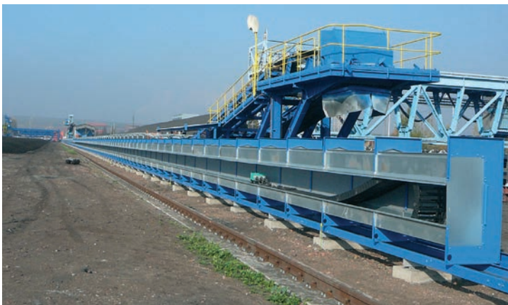
Longest igus® travel of 615 m with rol e-chain® and chainflex®-cables
