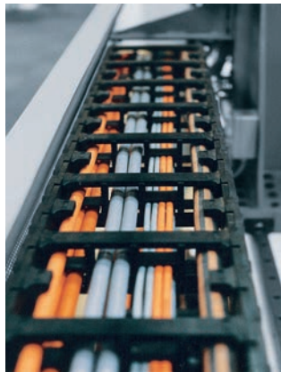
Orderly laid cables with igus® interior separation
