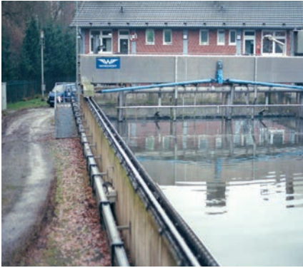
The scraper moves on the 38 m long final clarifier in round-the-clock operation. The energy supply is done via the lbt flizz® system
