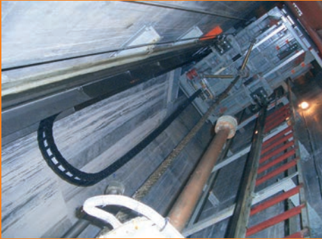
E2/000 - high stability in this elevator with an height of 160 m
