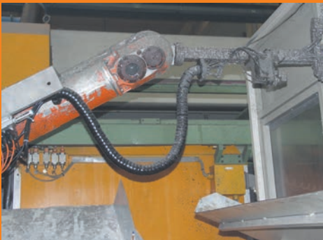
triflex® R in a magnesium die-casting industry (heat, dirt, oil, metal chips, dust, etc.) - failsafe
