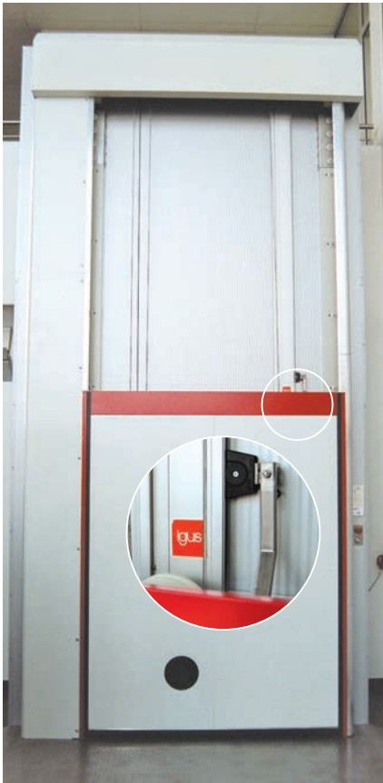
Energy supply to the strip at cold storage house doors, in operation for more than one year.
