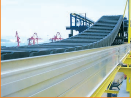
Seawater resistant super-alu-trough in a RTG-crane. Long travel with the E4 system
