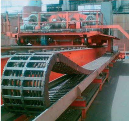
rol e-chain® Serie 5050R in a steel plant in india with highly corrosive atmosphere - s = 22\text{ m} , v = 1\text{ m/s} , a = 1\text{ m/s}^2
