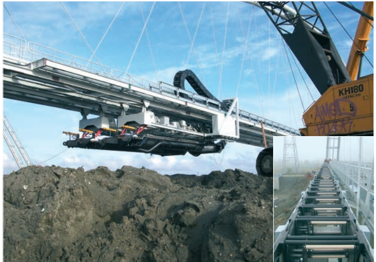
Cleaning of a port basin in Antwerp. On a stroke of 138 meters an e-chain® Series E4.350 guides cables and hoses with a total additional load of 98 kg/m
