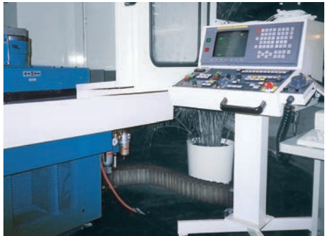
triflex® 332 as unsupported link from machines to control desk
