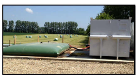
Citerne souple (stockage percolât)
