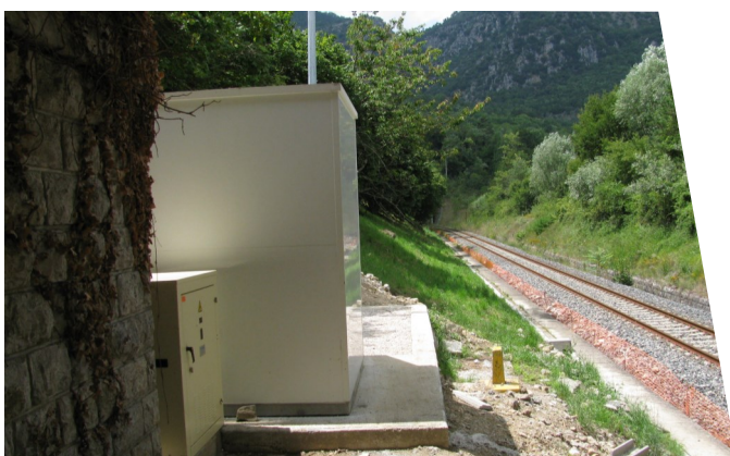
Tunnel de Braus, communication GSM-R
