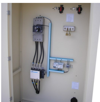
Compartment basse tension
