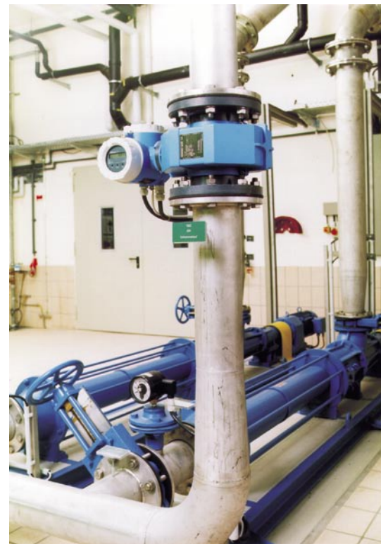
Sludge flow measurement with Proline® Promag electromagnetic flowmeter
